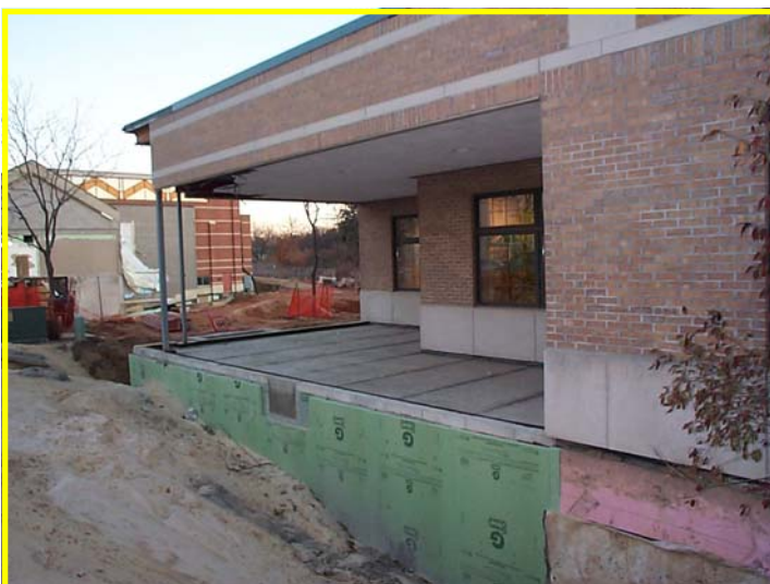
Northeast corner of the library. Constructing the Kenneth J. Mack Reading Room
